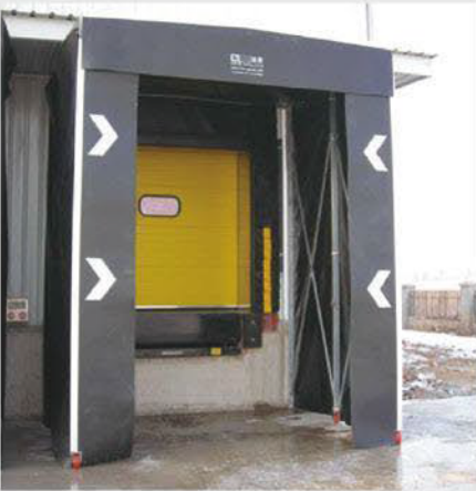
GMS Tunnel dock shelter
